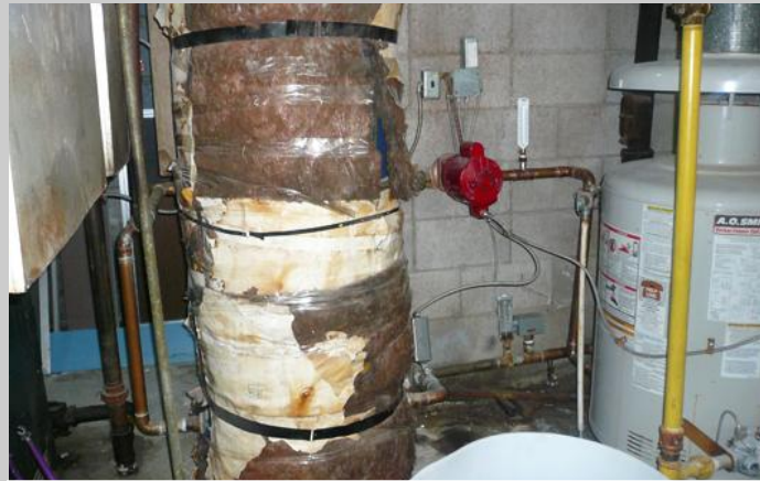
BOILER – 700 Ross St., Burlington
